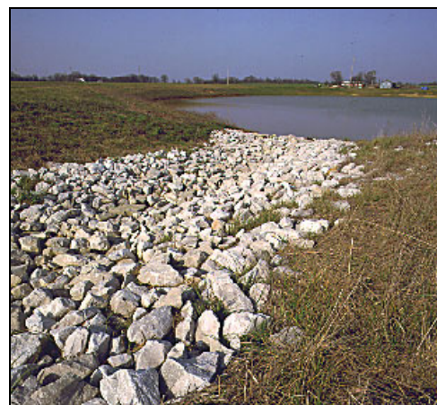
Rock Rip-Rap Sediment Control (Dept. of the Interior, Office of Surface Mining, http://www.osmre.gov/ocphoto.htm )
