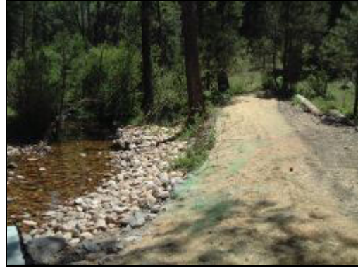
Rock Riprap and Jute Matting Erosion Control along a stream. (Photo: Lainie Levick)
