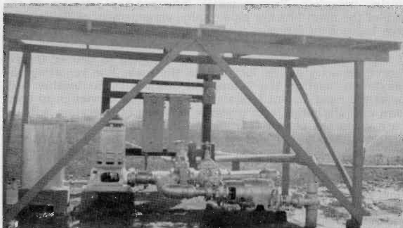
Plate XII.—Electric motor-driven centrifugal pump used as a booster with a deep well turbine for sprinkler irrigation near Tucson, Arizona.
