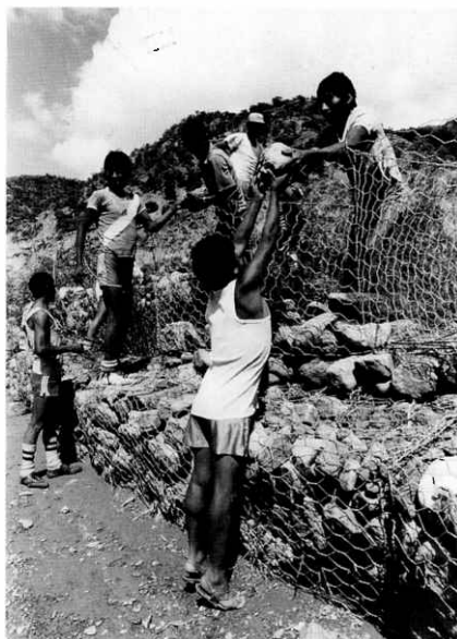
In Bolivia, project participants build stone gaviones to protect adjacent agricultural lands from flooding.
