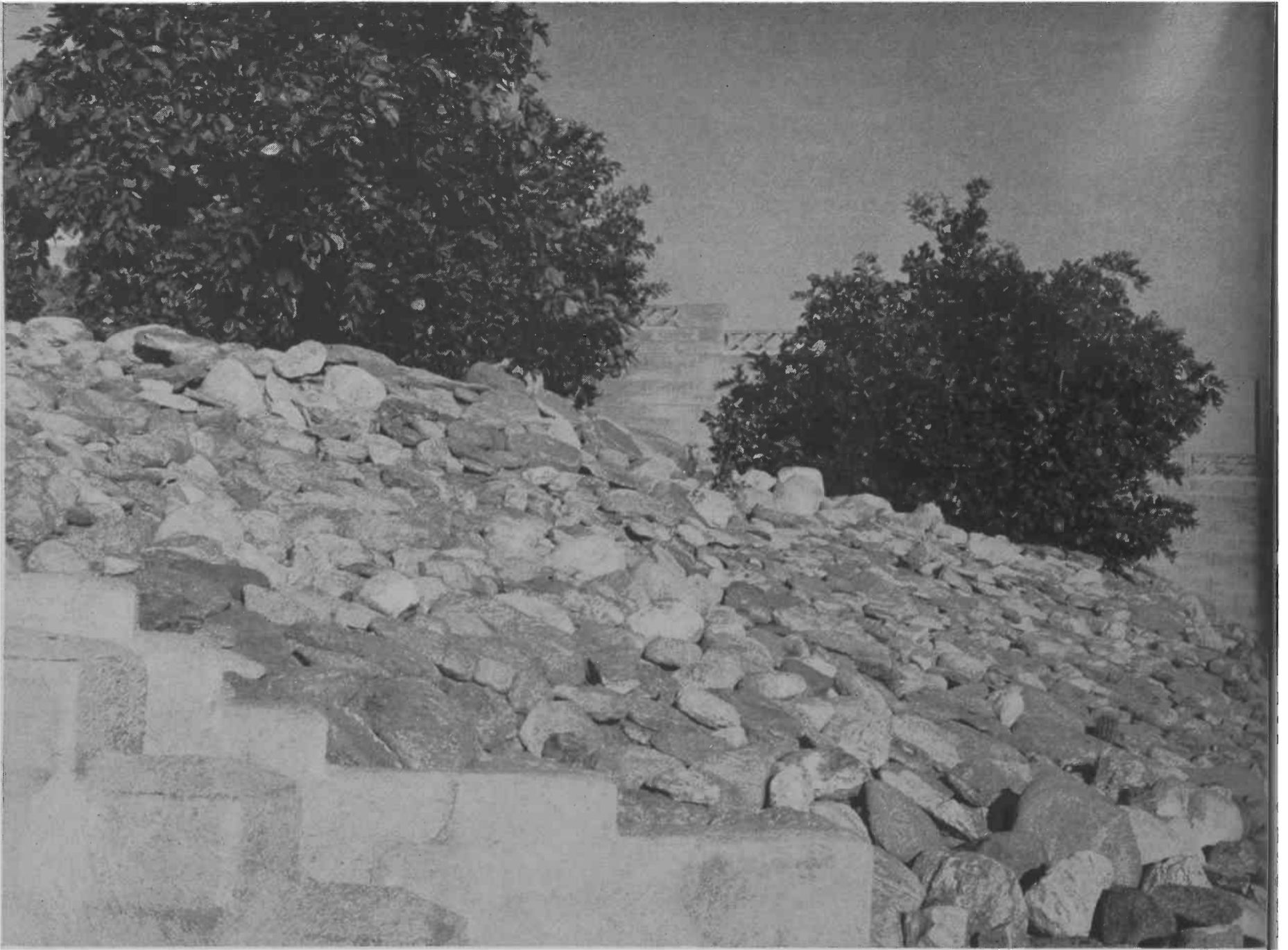
Figure 1. Rock mulch covering this patio slope in Tucson foothills is lain over soil which has been stabilized against wind and rain erosion since 1963.
