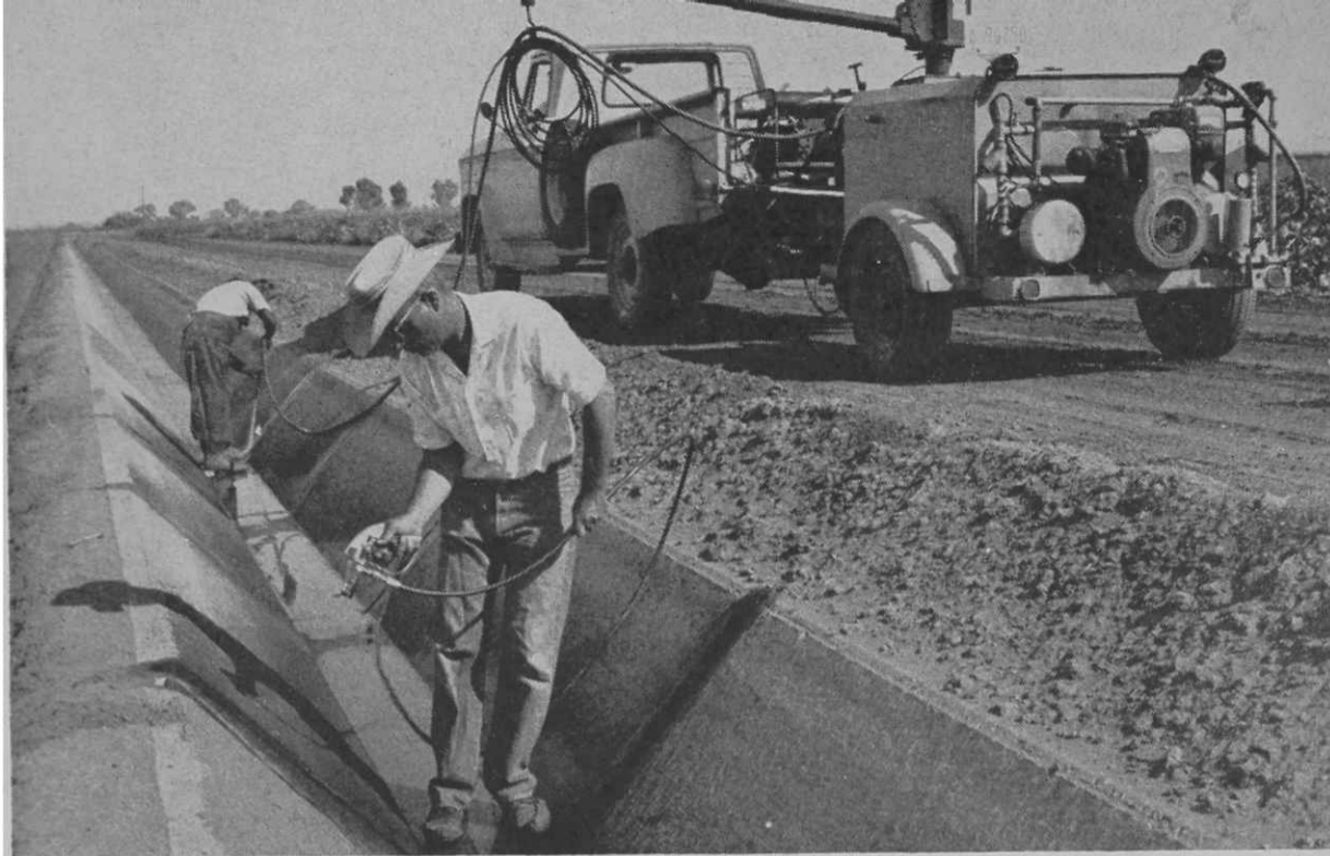
NEW DITCH SEALING technique is most efficient with a three-man crew. One ← man jets the cracks, one sprays on the sealer and third drives the truck.
