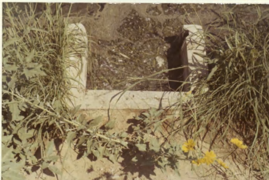
Figure 5. Enlarged view of drain gate showing a high amount of scum and organic matter.
