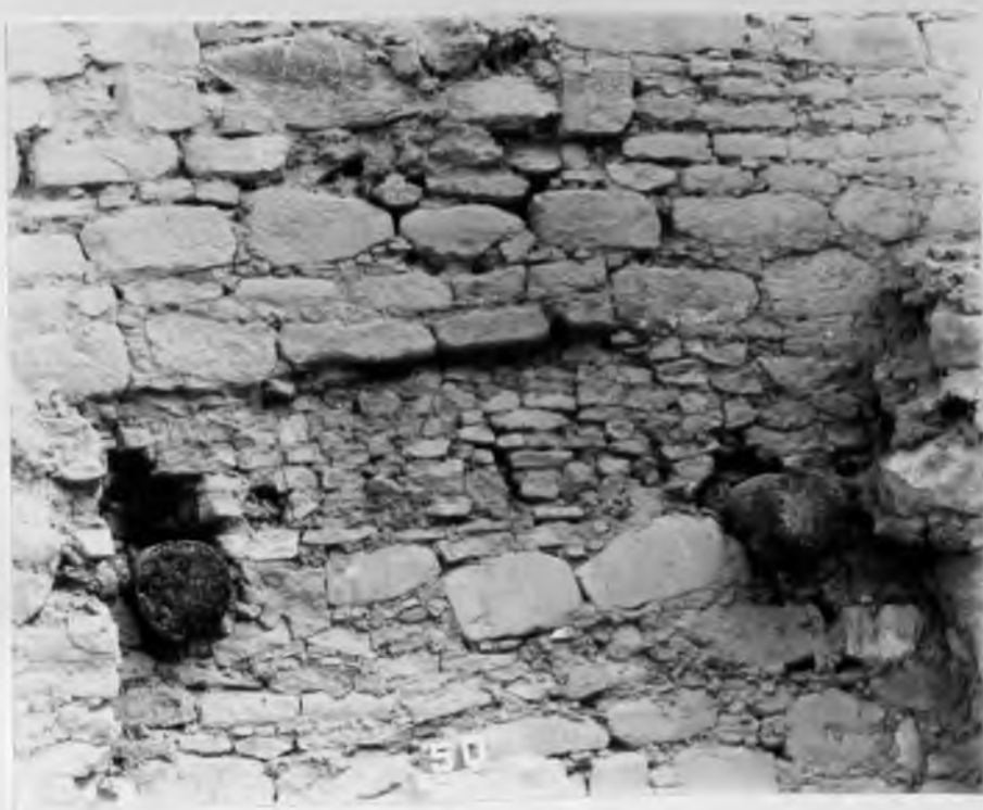
Plate III. South wall of Room 50 showing two first story beams in situ . Both timbers are dated at A.D. 1076c. (Courtesy National Park Service)
