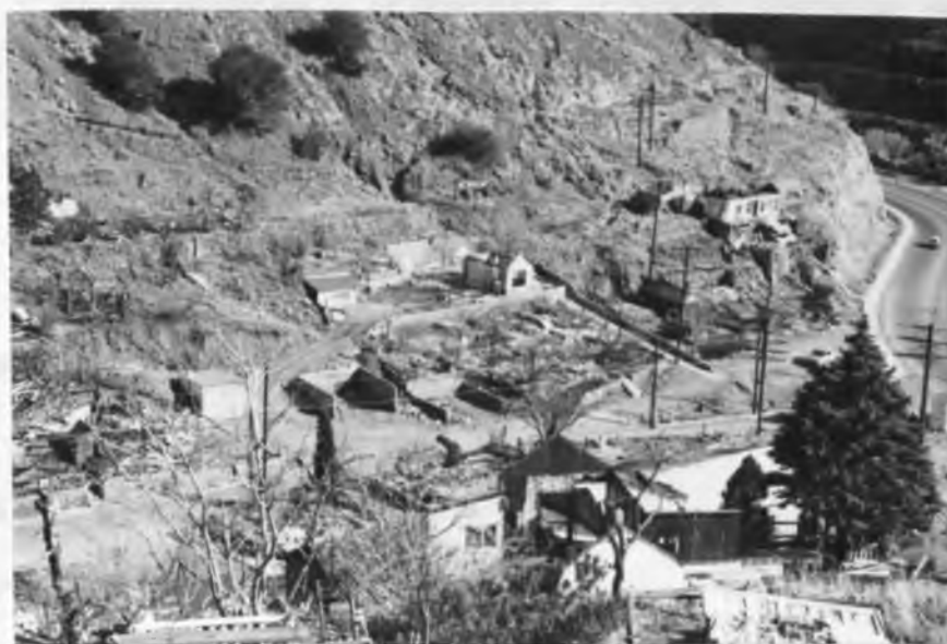
Figure 24. Houses being torn down to make way for the westward extension of the Lavender Pit.
