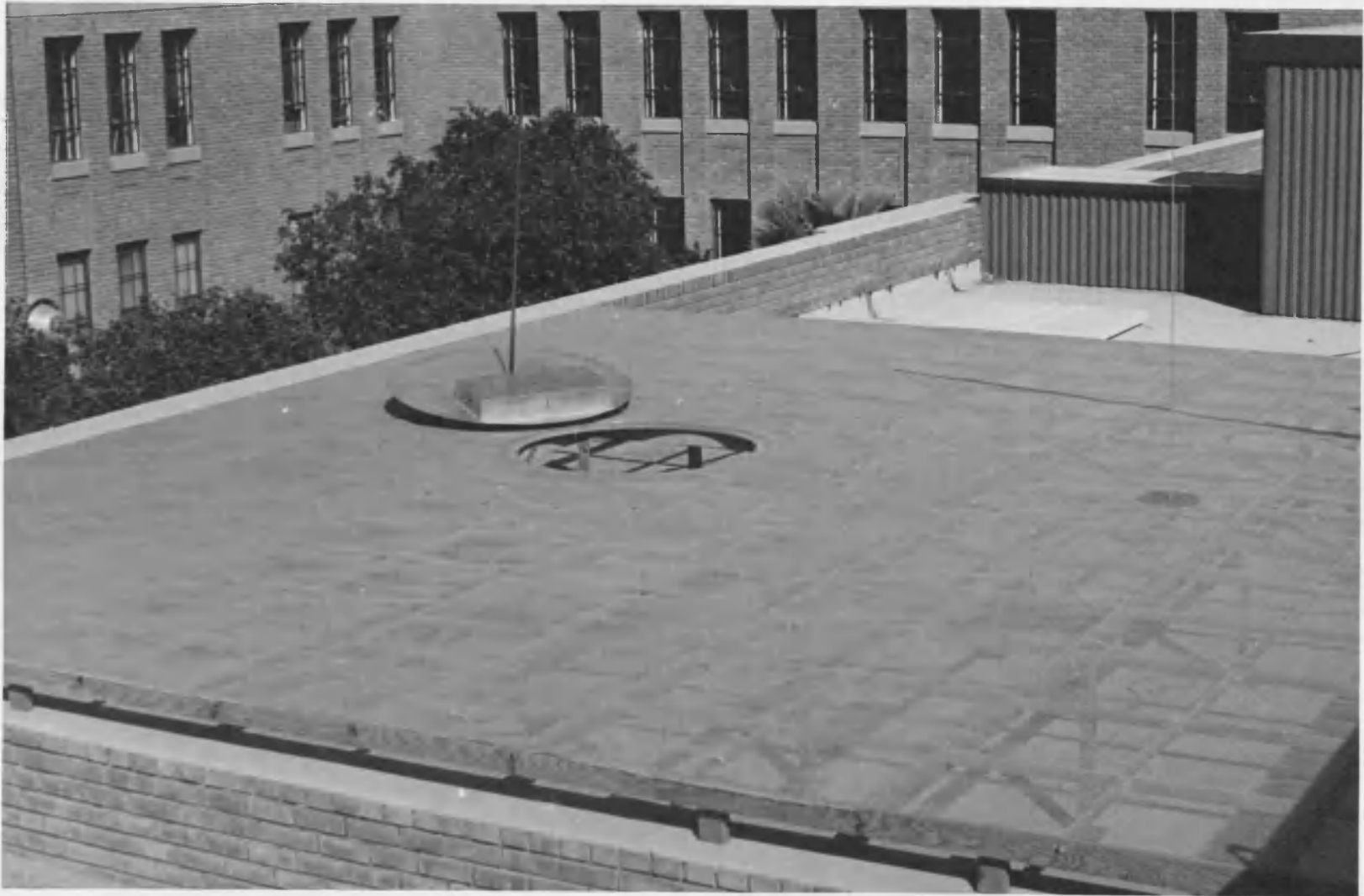
Fig. 2.4 Test Facility with Model Area Removed
