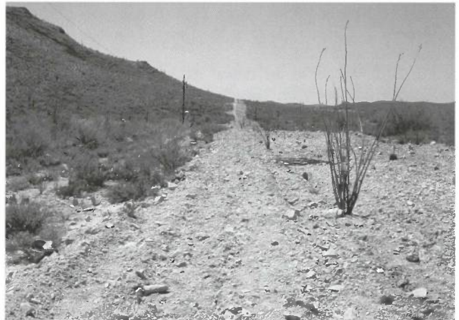
Figure 10D. (June 3, 2004) The new pipeline was installed a few months before this match. The ocotillo in the right foreground was one of several of these plants that were salvaged and planted along the pipeline corridor (R.M. Turner, Stake 905A).
