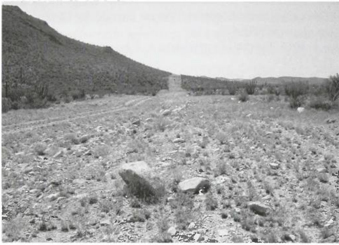
Figure 10A. (September 1958) Southerly view of a newly installed pipeline for transporting gasoline from El Paso, Texas to Tucson and Phoenix. It crosses the western edge of Tumamoc Hill on an easement through the Desert Laboratory property. The vegetation present is mostly annual forbs and grasses (R.R. Humphrey).
