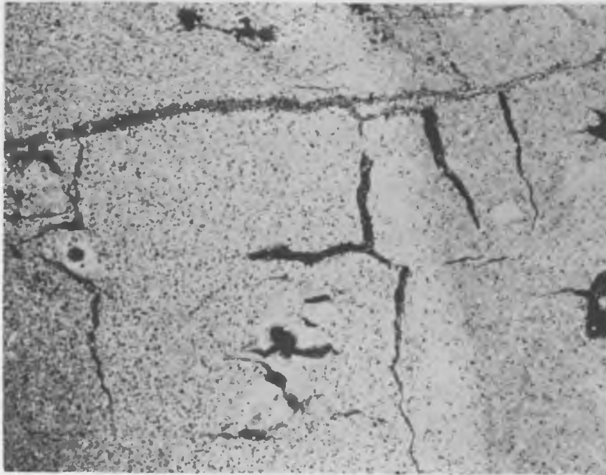
Figure 24. Photographs of Dessication Cracks. 14.4X
