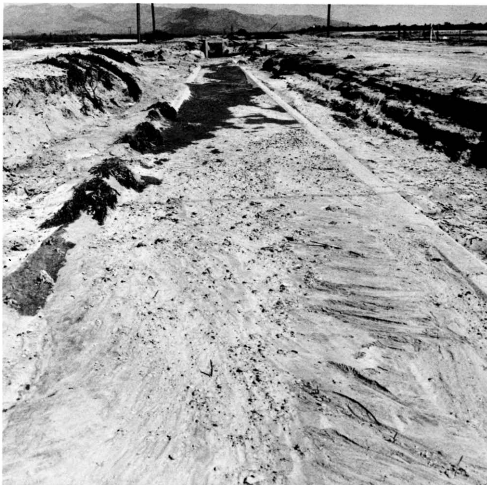
FIGURE 17. IRRIGATION CANAL FILLED WITH SAND AND SILT IN THE ROOSEVELT IRRIGATION DISTRICT (COURTESY USDI BUREAU OF RECLAMATION).
