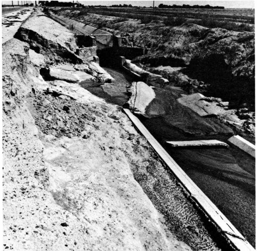
FIGURE 18. STRUCTURAL DAMAGE TO IRRIGATION CANAL SYSTEM IN THE ROOSEVELT IRRIGATION DISTRICT (COURTESY USDI BUREAU OF RECLAMATION).
