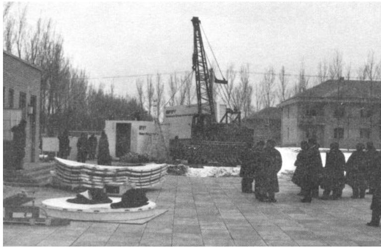
Figure 2 - Shelters and Antenna Before Assembly
