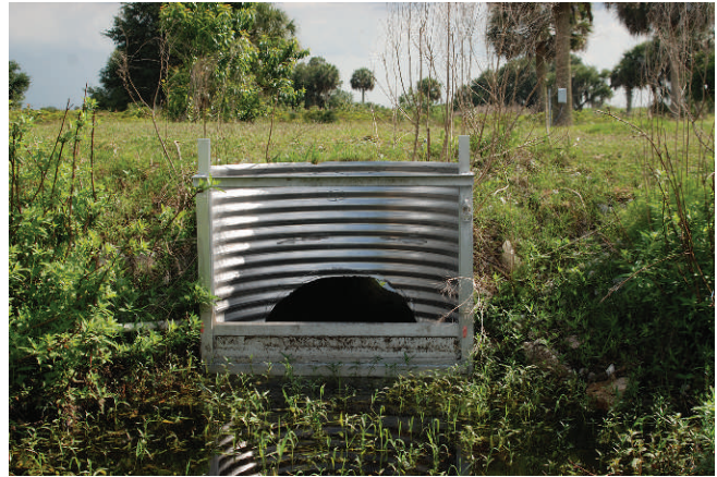
Figure 1. A culvert with a riser board installed to retain water. Note the padlock on the right is included as one element to ensure contract compliance. Photo courtesy of Elizabeth Boughton.
