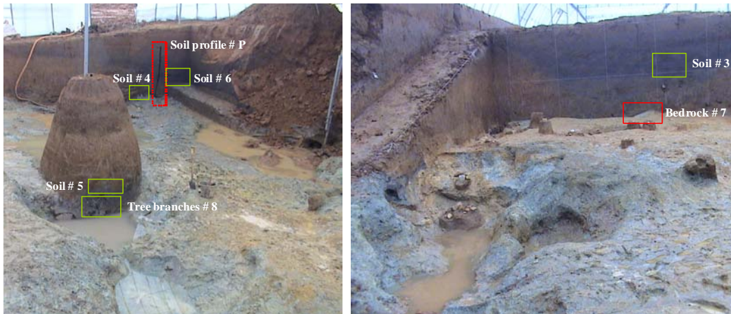
Figure 3 Photographs of the west side of locality 12 showing (left) the locations of sample spots 4, 5, 6, and 8 (highlighted in green) and soil profile #P (highlighted in red) marking the location of the soil profile in Figure 2; and (right) sample spots 3 and 7 on the east side of locality 12.
