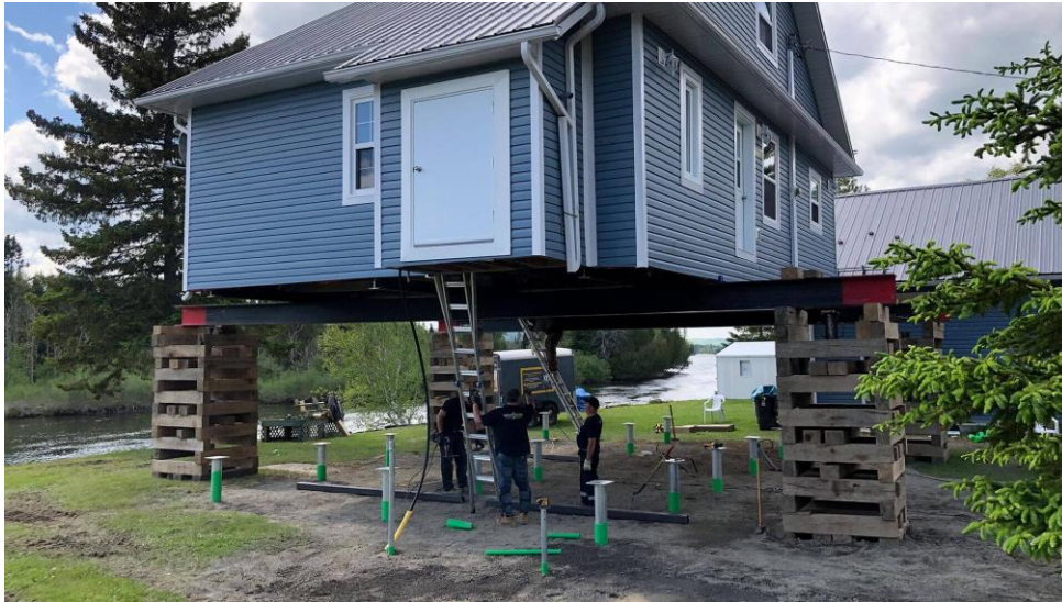
Figure 2. Existing home near a river being lifted to install a higher helical pier foundation to adapt to increased flooding.
