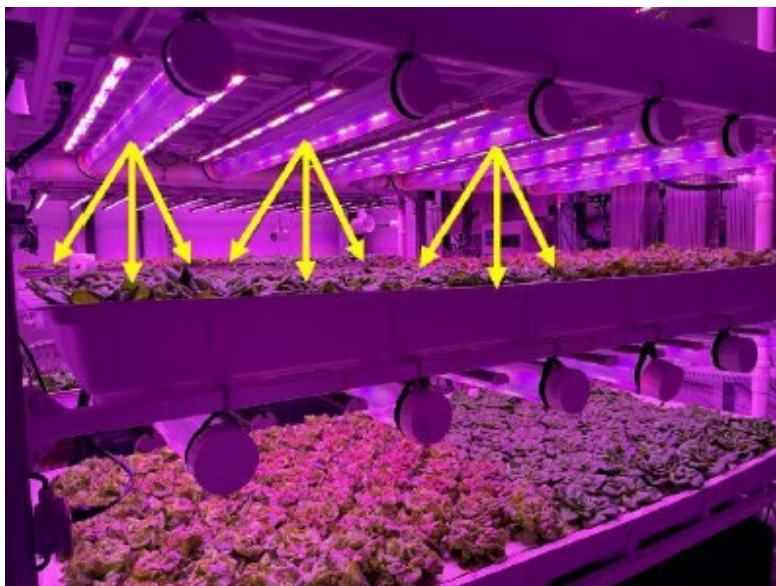
Figure 10: The vertical airflow system installed within the growth chamber.
