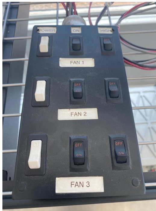
Figure 15 Scrubber fan controls and settings
