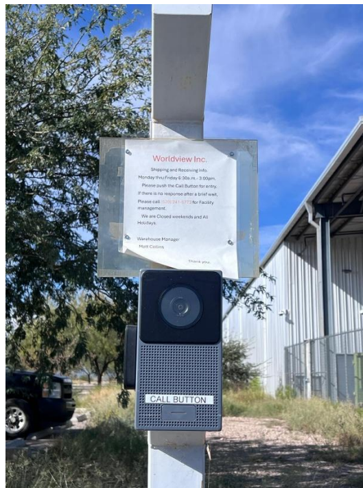
South gate call system. Reads, "Push call button for entry, if there is no response after a brief wait, please call 530-241-5773 for facility management"
